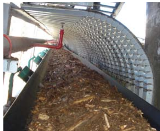
Biomass transported to the boiler of Pacífico Mill
